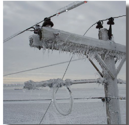
Ice that accumulates on lines and strong, high winds can impact distribution.
