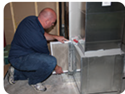
Air filters should be changed regularly because the air inside our homes is full of particles.
